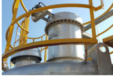
Silo Top Jet Filter
