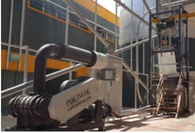
Pneumatic Conveying Systems
